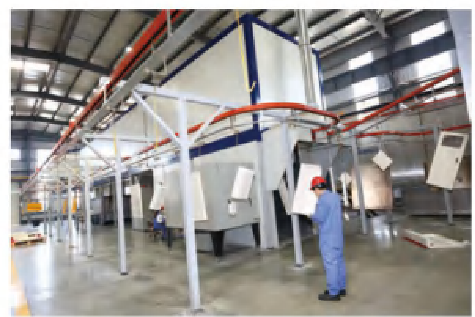
Automatic powder coating lines
